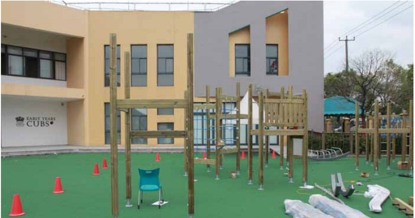
Our new primary playground equipment has arrived from Europe and construction has already begun. Look out for pictures and an update in next week's newsletter...
